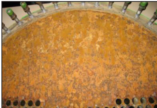
Shows extensive corrosion of the metal on the tube sheet and the end cover
